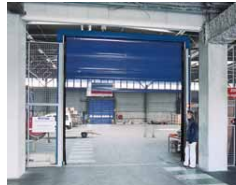
Automatic rapid shutter door, hangar, LYS
