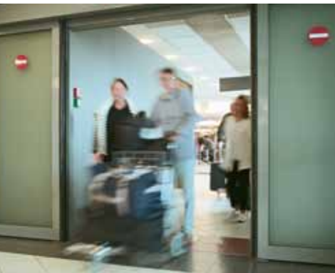
Automatic fire protection door, baggage claim, LYS
