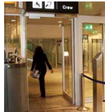
Revolving door operator, crew entrance, ZRH
