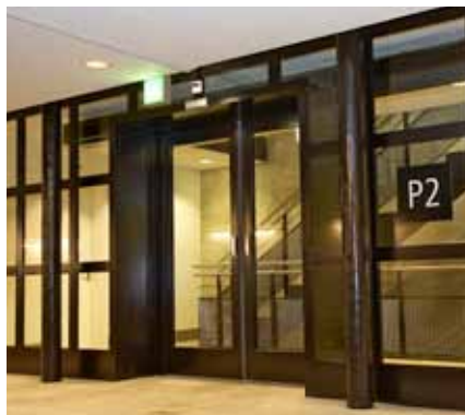
Automatic smoke-protection door, multi-storey car park
